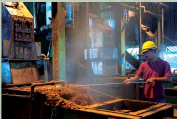
Solvent extraction plant at Keningau mill
